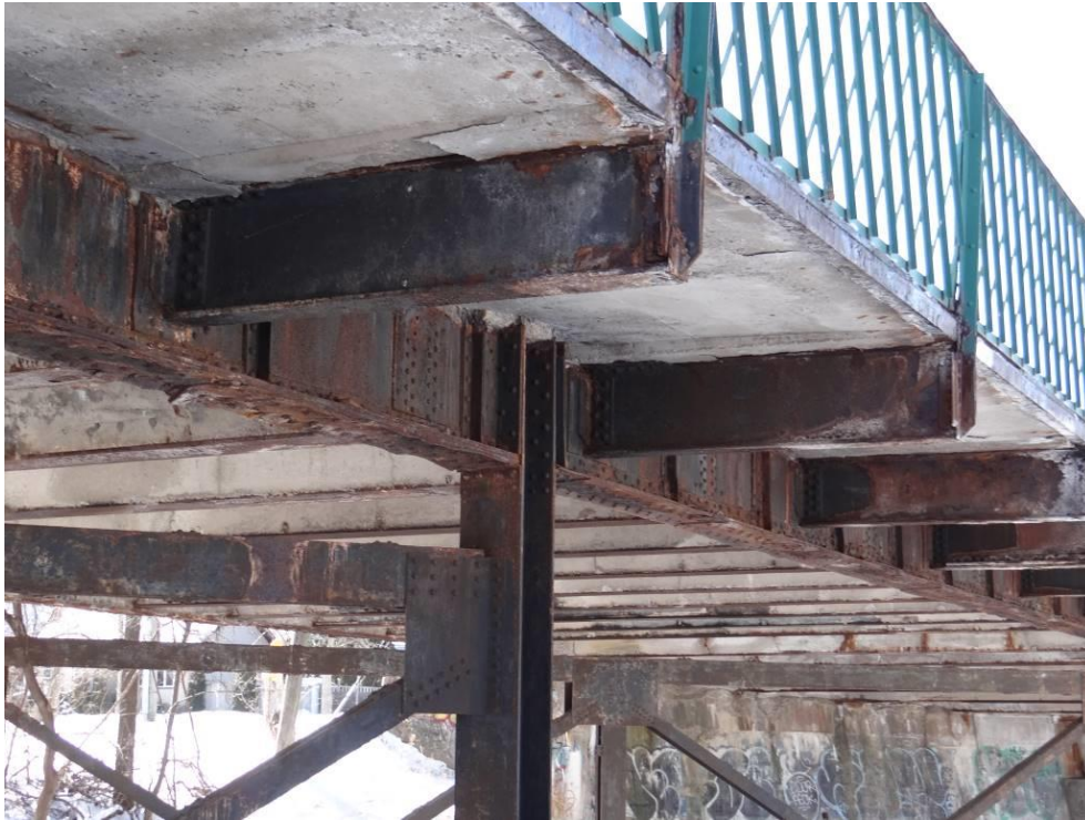
Plate 7: Bridge soffit showing lower portion of riveted through-plate girder and transverse stringers supporting the concrete sidewalk, looking southwest.
