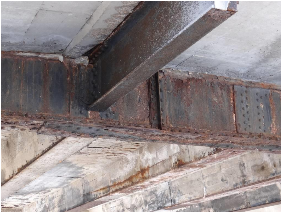
Plate 10: Detail of connections between steel plate girder and transverse stringers, looking south.
