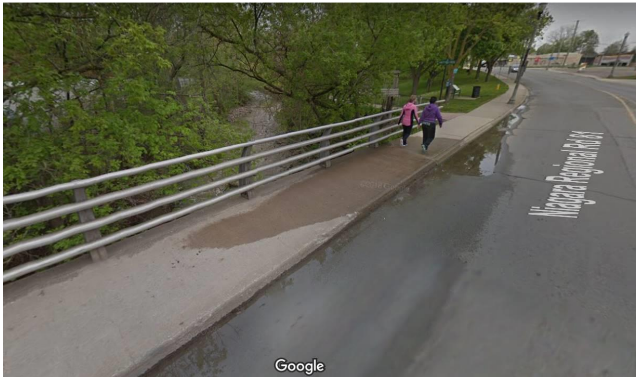
Figure 13: Forty Mile Creek Bridge, Main Street West, Grimsby, built in 1922 (Google Streetview)
