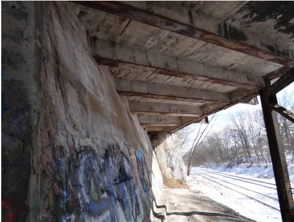
Plate 11: East abutment and soffit of eastern span. Note the skew of the structure.
