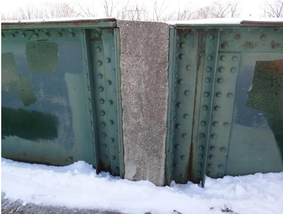
Plate 21: Detail of concrete pillar at deck level that integrates the steel plate girders to the bents.
