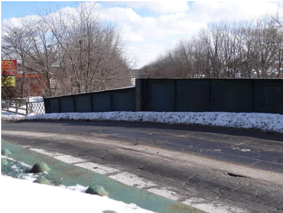
Plate 18: East span of the bridge at deck level, looking south. Note the steep slope of the approaches.
