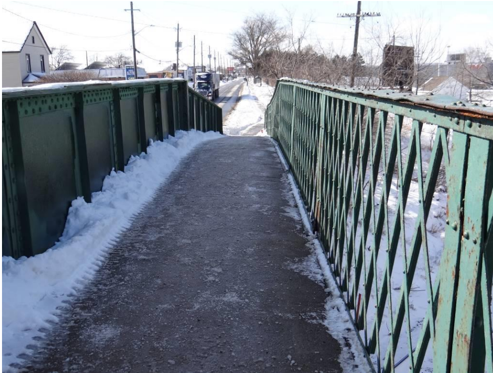
Plate 19: Northern pedestrian sidewalk, looking west from the center span. Note the riveted steel plate through girder at left and steel lattice railing at right.
