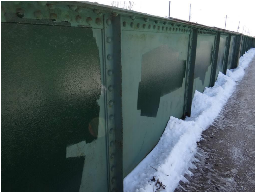
Plate 20: Detail of north riveted steel plate through girder at deck level, looking southwest.
