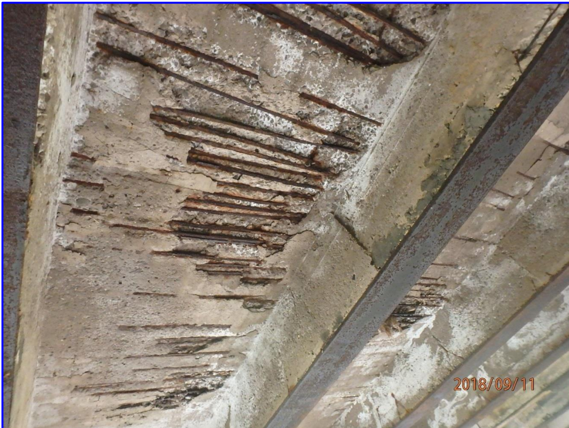
Photograph 6 – Deterioration in concrete bridge deck soffit (typical)
