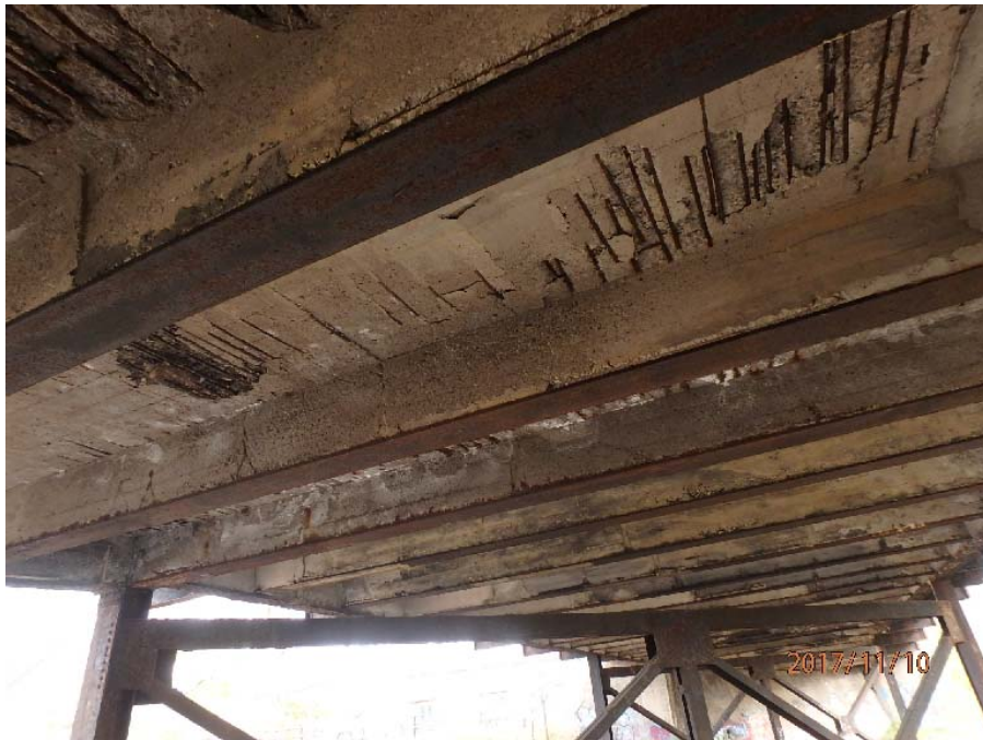
Photograph No. 2: 0465: Very severe concrete spalling on bridge deck soffit.
