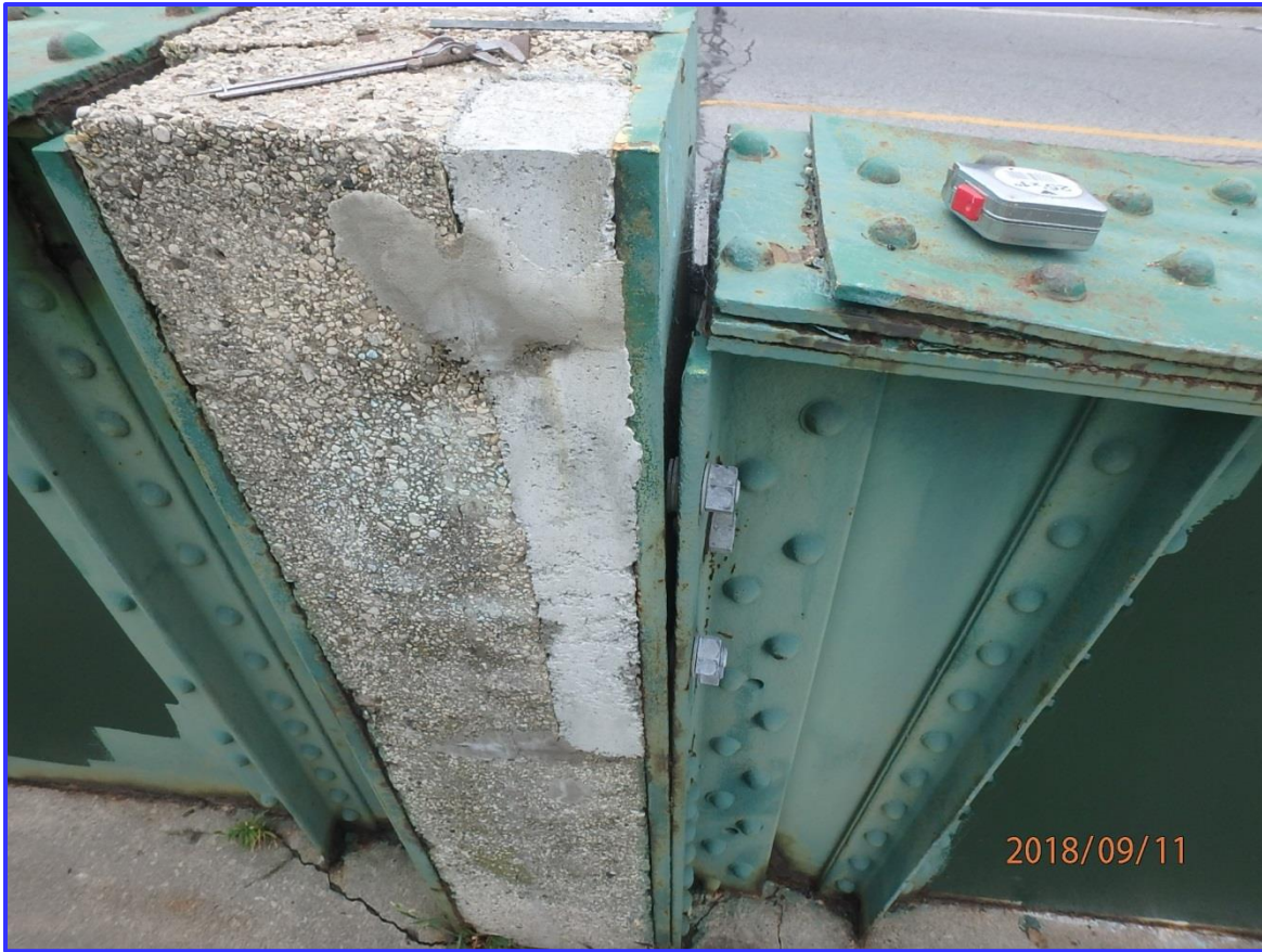
Photograph 3 – Failed rivets and separation of girder at northwest pier column
