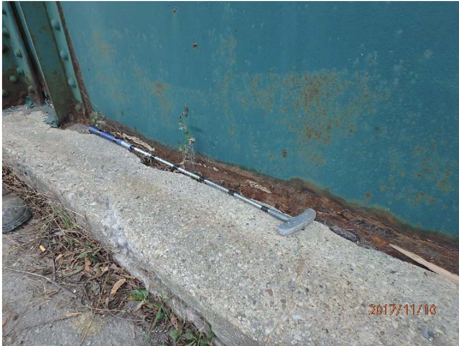
Photograph No. 3: 0430: Perforation in the through-plate girder web
