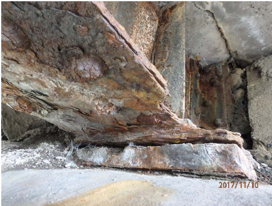
Photograph No. 4: 0541: Section loss of the bottom flange of the through plate girder at the south east bearing
