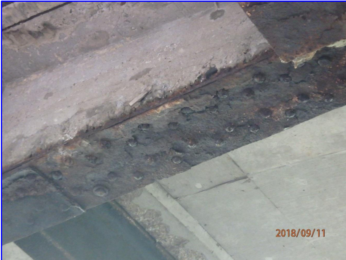
Photograph 5 – Severe corrosion on underside of main girder bottom flanges
