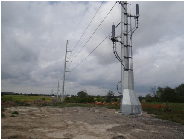
Plate 7: Wind turbine infrastructure on the north of the study area, looking northwest.
