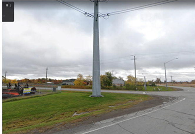
Transmission Pole located on Regional Property (NE corner)
