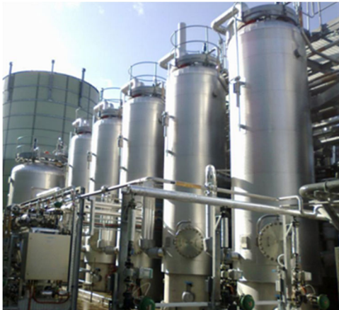
Figure 2-1 THP system at Davyhulme, UK
