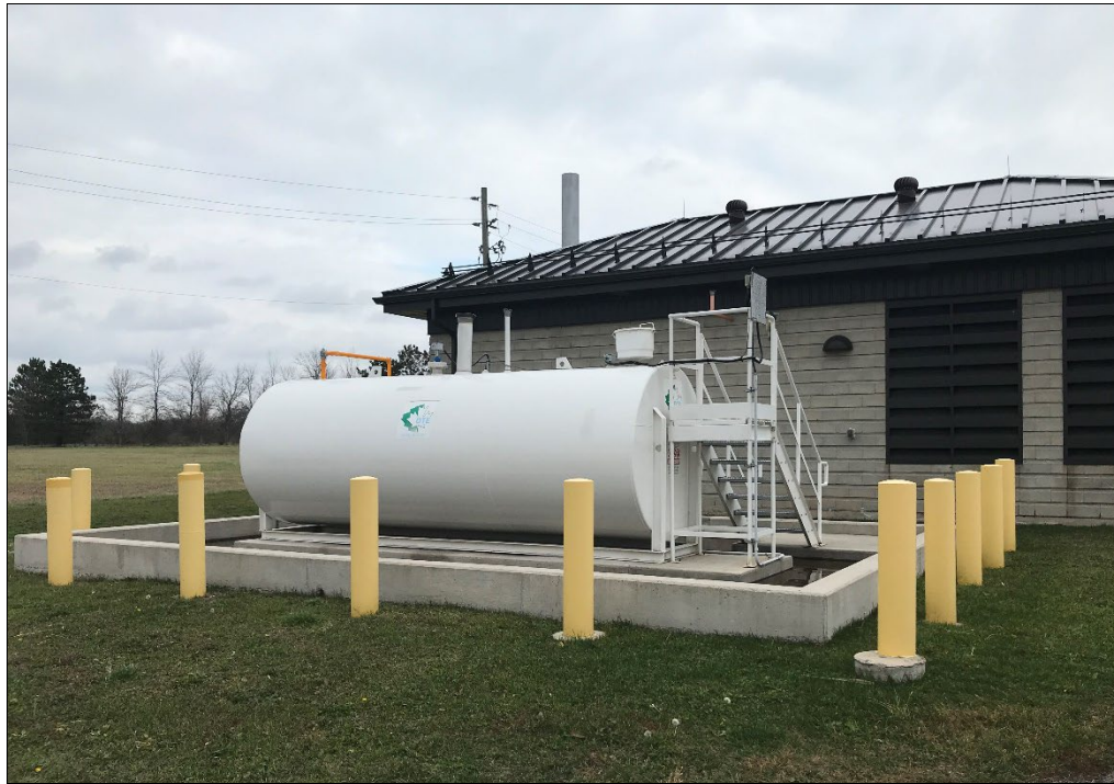
Photo 11: Diesel fuel AST located at the South Side High Lift Sewage Pumping Station.
