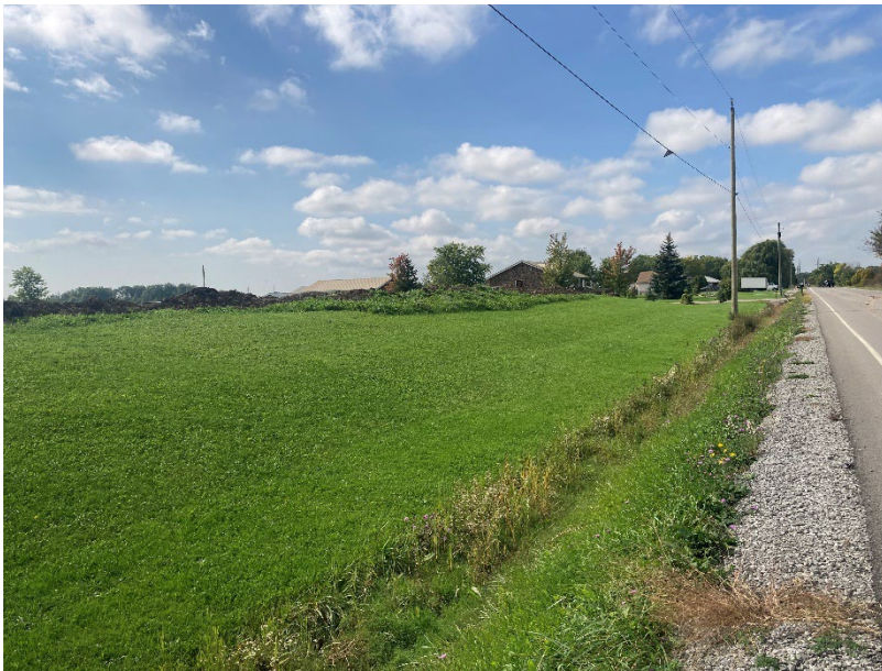
PHOTOGRAPH 10 View of Barron Road facing west. Also visible is the roadside culvert/ditching.
