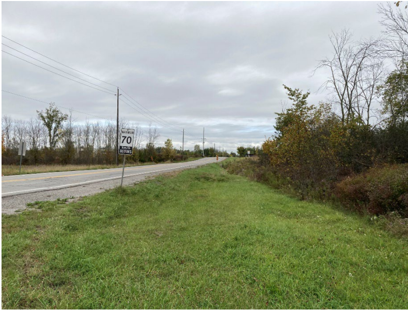
PHOTOGRAPH 15 View facing northwest of Montrose Road from Reixinger Road. Note the minimal roadside ditching.
